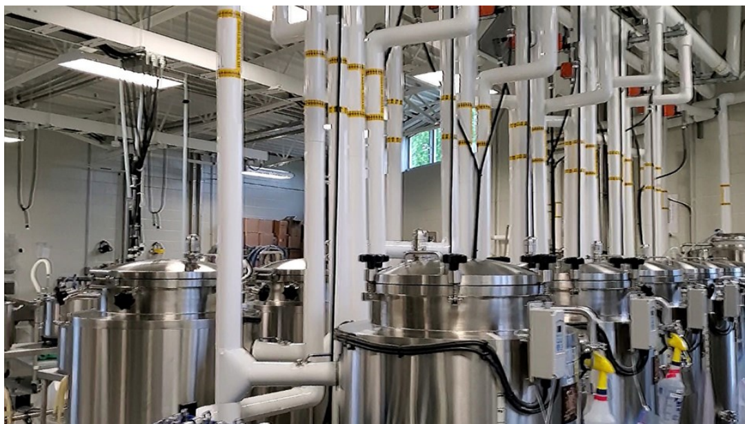
Photo: New glycol lines in the KPU Brew Lab brewery as part of the renovation/upgrades in 2020.
