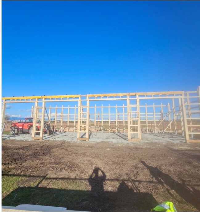
The picture above is of the new shed, Garden City lands, Richmond, courtesy of Alysha Felder
