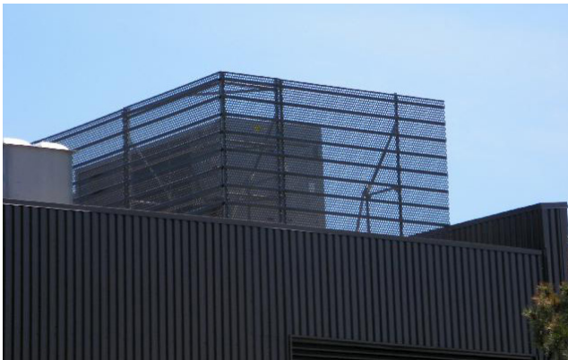
Above - Screened mechanical systems
