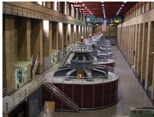
Figure 11.22 Hydroelectric generators at the Hoover dam. (credit: Jon Sullivan)
